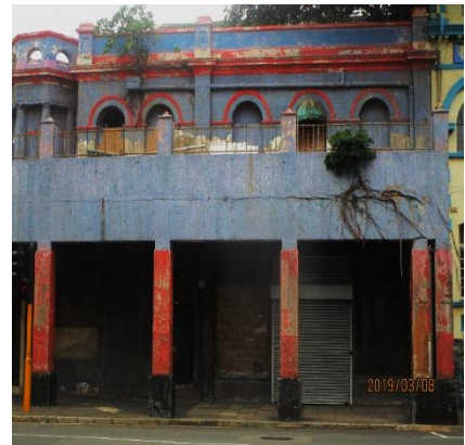
Bad buildings in Durban. SOURCE: eThekweni Municipality, 2020
